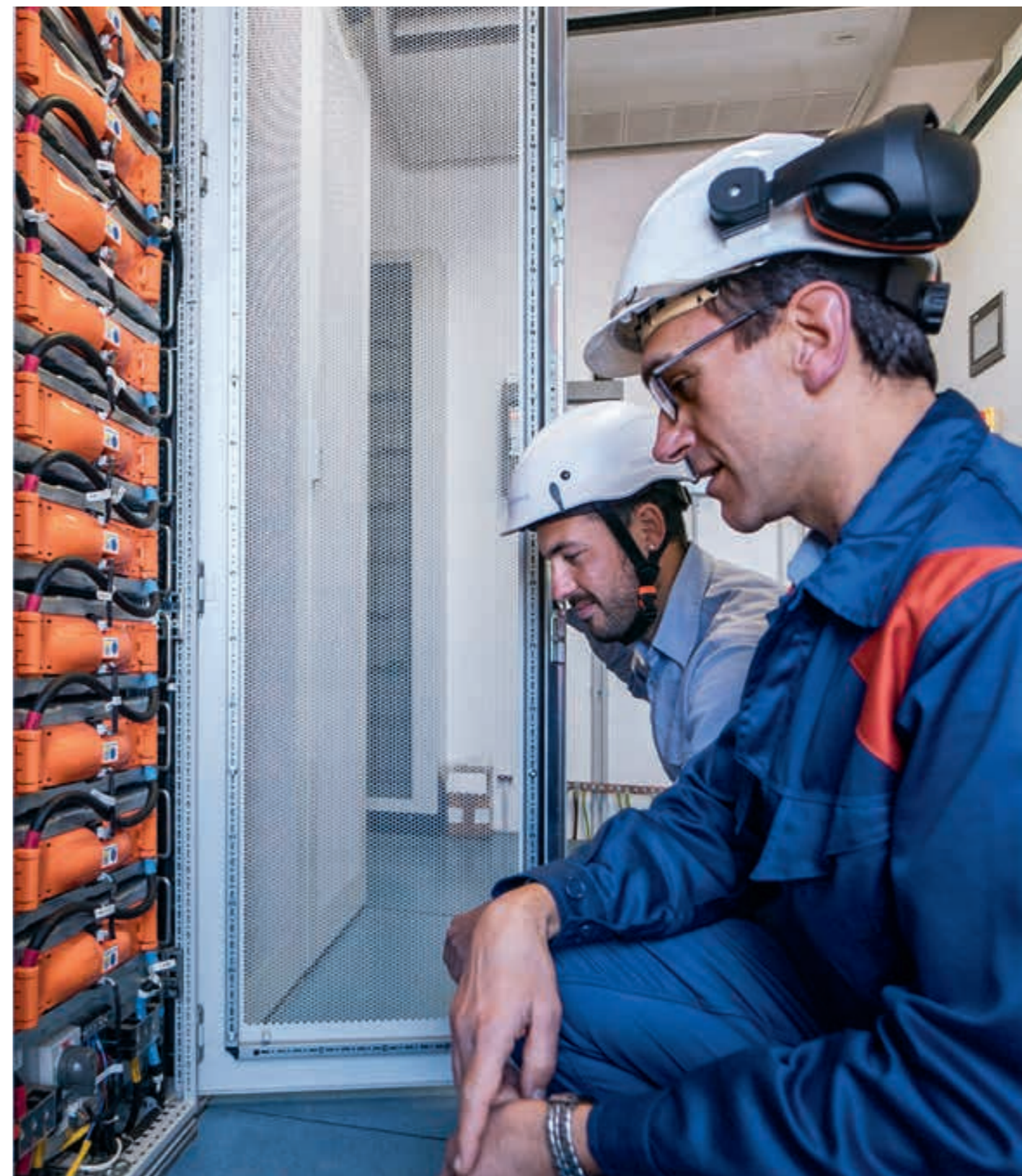
Enel technicians maintain Ventotene’s energy system, ensuring a reliable and sustainable power supply for islanders.
