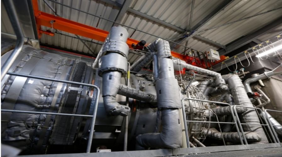
"Anna", the SGT-800 gas turbine, can generate up to 57 megawatts electrical energy.
