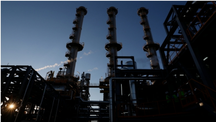
Each of the three SGT-800 gas turbines has its own chimney and bypass stack.
