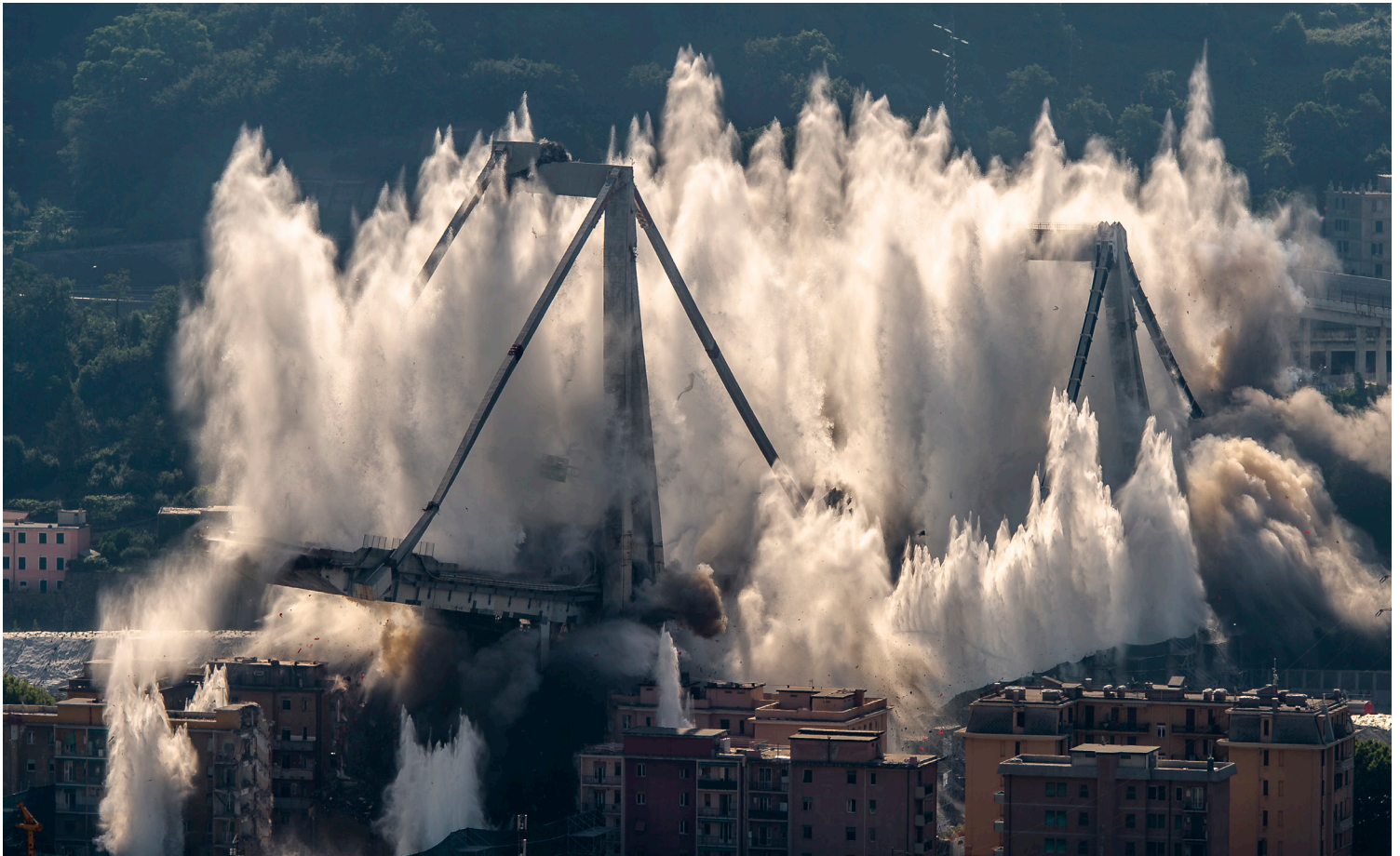
Remains of the old bridge had to be demolished for the construction of the new one
